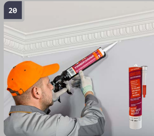
20 Using Europlast Multipurpose adhesive fill the spaces in the junction area between the cornice and the walls/ ceiling, where the adhesive has not shown on a surface.
