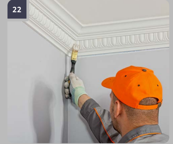
22 Paint the cornice following the instruction of paint producer, starting from the corners of the elements (room).
