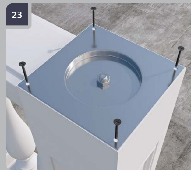
23 Secure the flange on the newel with a nut and self-tapping screws.
