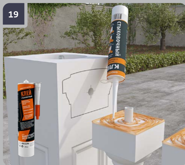
19 Apply Evroplast for Bonding joints onto the top (adjoining to the handrail) sides of the balusters.
