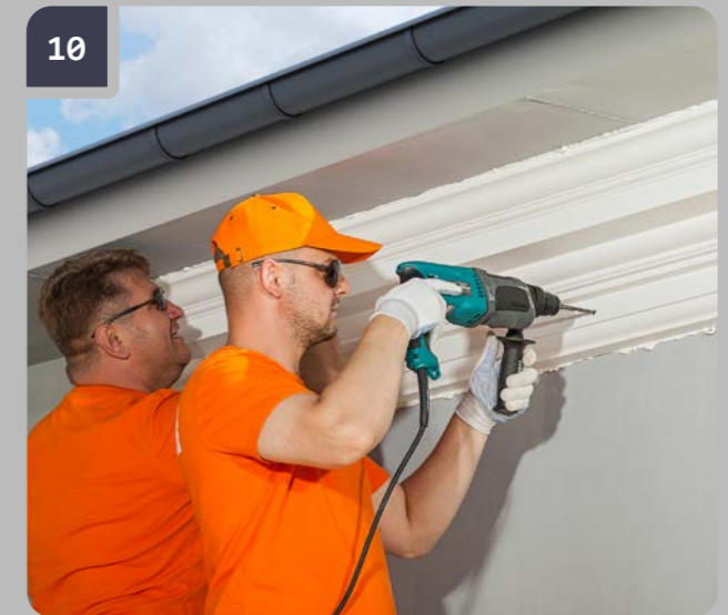
10 Use a perforator to make holes for impact anchors spaced at ~600 mm.
