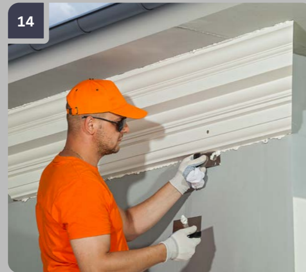
14 Immediately after putting in the self-tapping screws remove excess adhesive with a palette knife.
