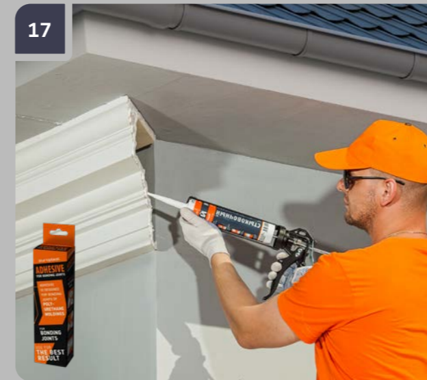
17 Put the «Evroplast for bonding joints» Adhesive on the free end of an already-mounted item.
